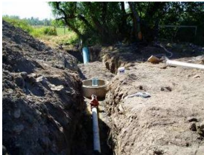
Construction underway of irrigation pipelines in Clallam County that replace older, less efficient irrigation ditches and save water in the over-appropriated Dungeness River.
