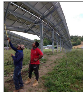
Figure 7: Raised Array at Maple Ridge Meats. Source: ruralsolarstories.org
